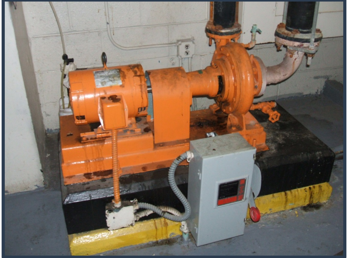
Base Mounted Hot Water Pump to AHUs (from boiler or heat Exchanger – usually insulated but some may not)
