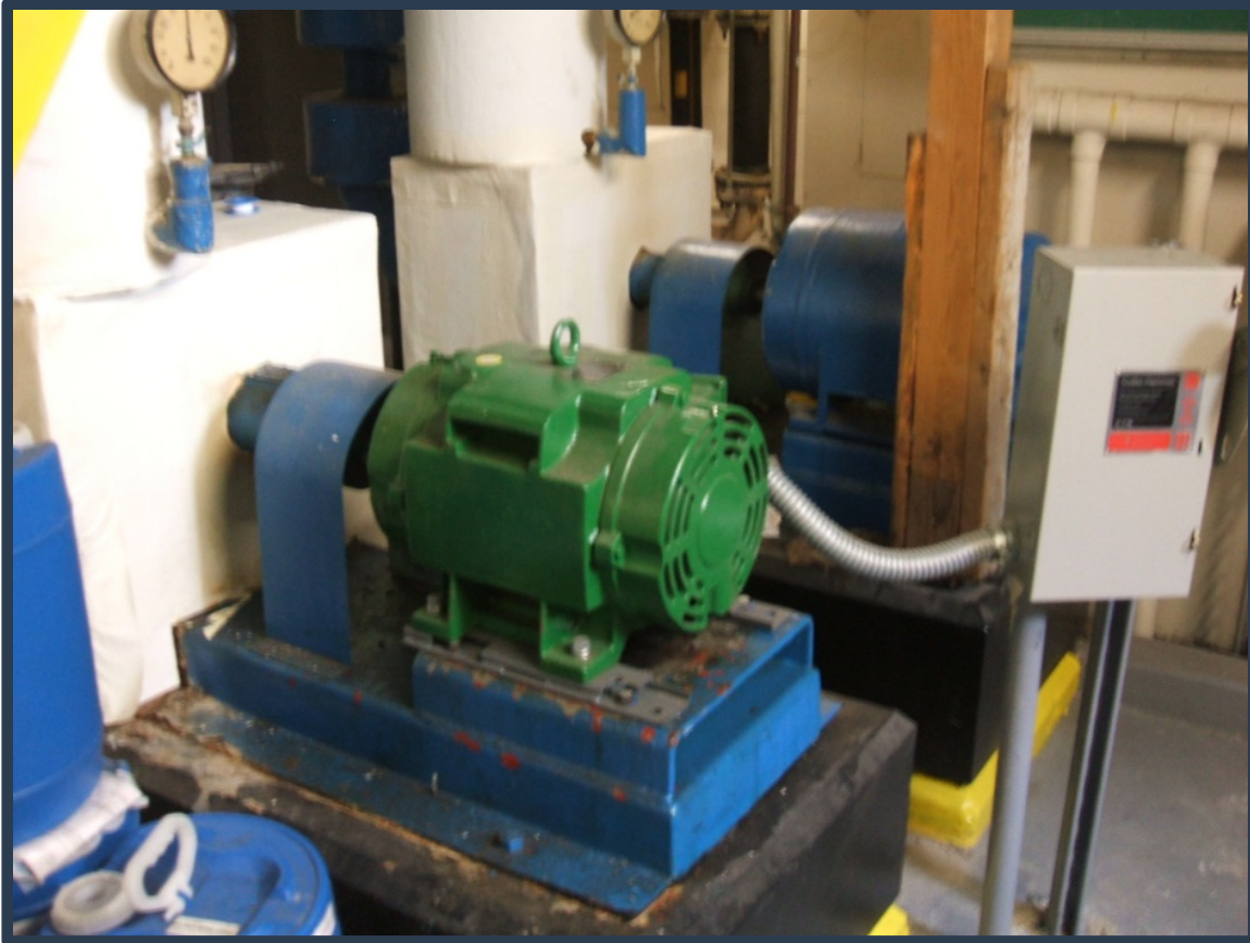
Base Mounted Chilled Water Pump (Chilled Water Pumps usually insulated; Condenser water pumps are not)
